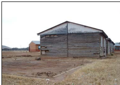
Collapsed classroom, Sibuyele Combined School
